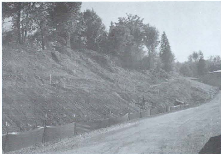
The first phase of the Des Moines Creek Trail is being carved on a hillside next to the sewer treatment plant. The trail will run from S. 200th St. to Des Moines Beach Park.
